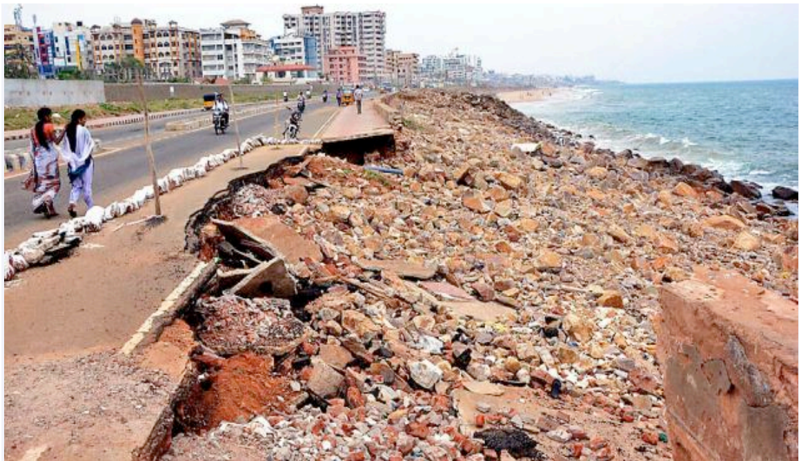
The Hindu The road washed-away near the fishing harbour left unrepaired, even after a month of Cyclone Hudhud leaving a trail of destructions in Visakhapatnam. Photo: C.V. Subrahmanyam
