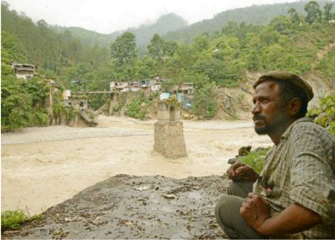
The bridge over Pindari river at Narayan Bagar village which got washed away during the recent flash floods in Uttarakhand. Photo: V.V.Krishnan
