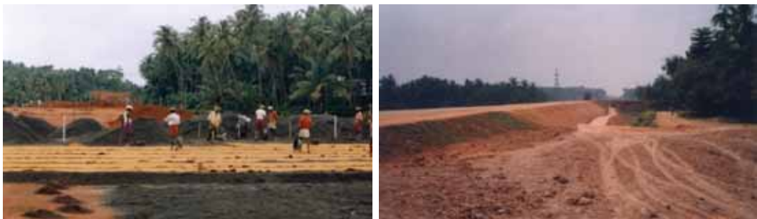
Laying of coir needled felt and Stabilized clay embankment, NH Bypass, Kozhikode
