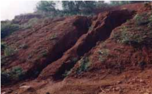
Eroded embankment of road embankment of road
