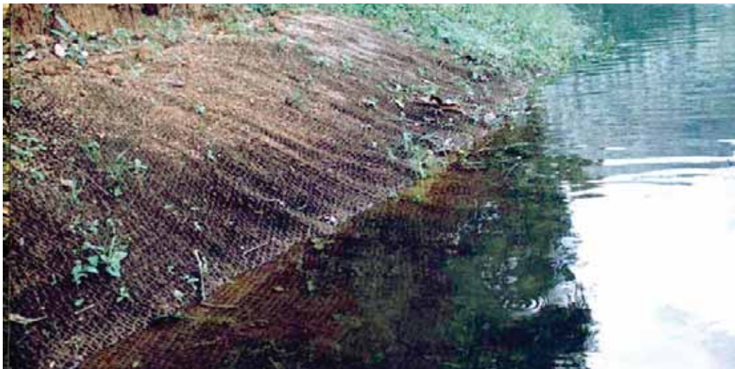
Protection of Periyar river bank
