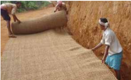
Keep the rolls adjacent and find out the overlap that can be given
