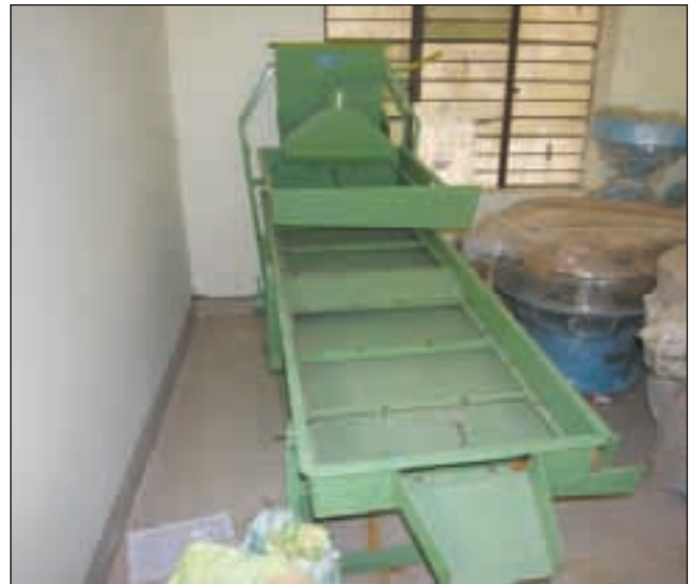
Grader installed in PPU
